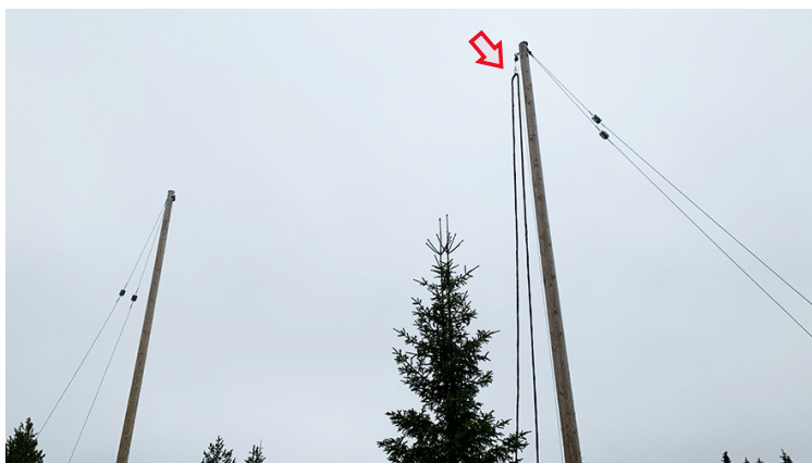
Figure: North-South antenna after lightning hit the left mast.
